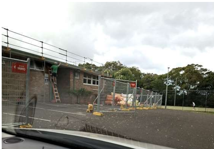
The roof coming off the Community Hall (Research Centre) (photo: Jennie Fairs)
